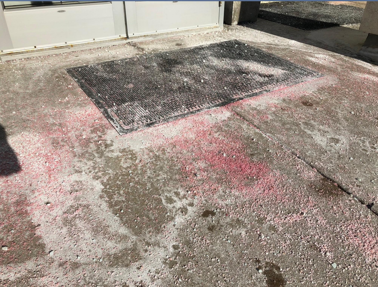
Incorrect Application Rate
